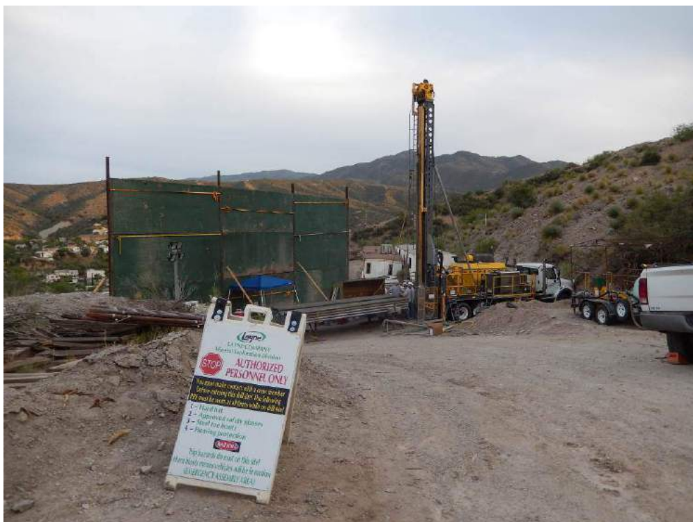
Plate 10-1 Large Sound Barrier Erected to Reduce Impact of Drilling for Local Residents, Hole VD14-01
