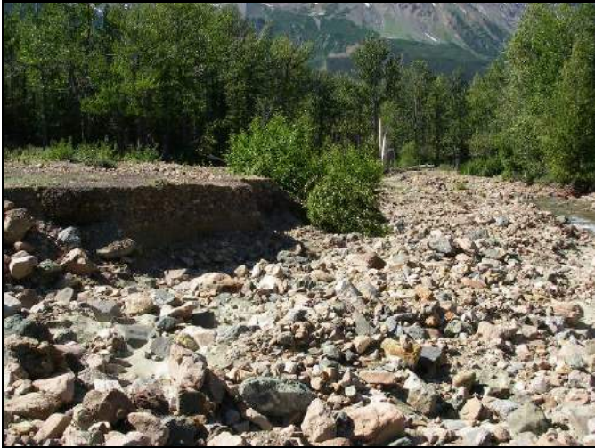
Site 180 – Downstream fresh erosion
