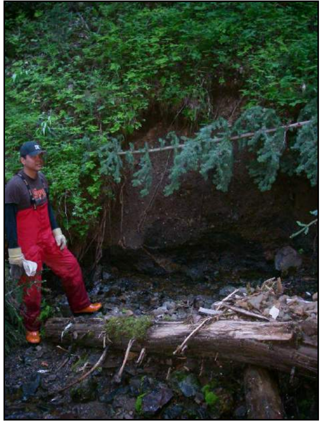
Site 173 – Upstream slope failure
